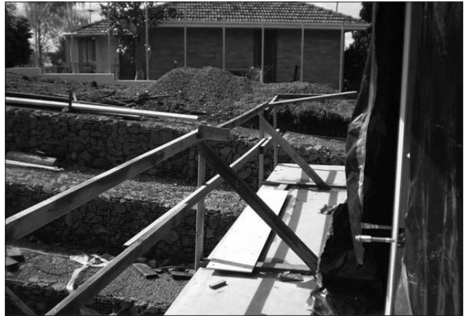
Wilkins Construction Pty Ltd wins lots of government school projects — but the standards of their safety on this Mount St Canice redevelopment in Sandy Bay leaves a lot to be desired. Poor quality handrails offer poor fall protection, plus hazard risk on the deck.
