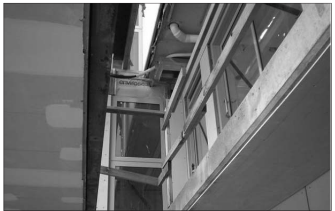
Poor quality handrails provide inadequate fall protection. No kick boards.
