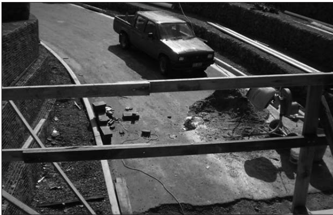
Poor quality handrails provide inadequate fall protection.
