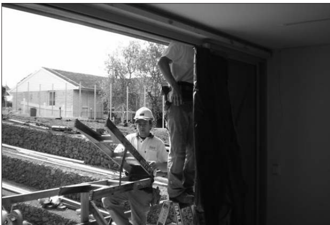
Worker standing on top rung of step ladder has no fall protection at all, as well as breaching AS/NZ standards for portable ladders.
