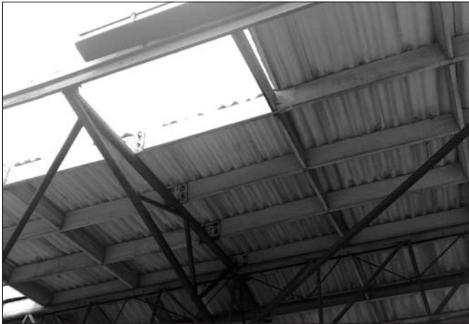
This photo was taken at the TCA football/cricket ground owned by Hobart City Council. The asbestos roof has broken edge with fibres visible. Workplace Standards approached HCC about the issue. Result unknown.
