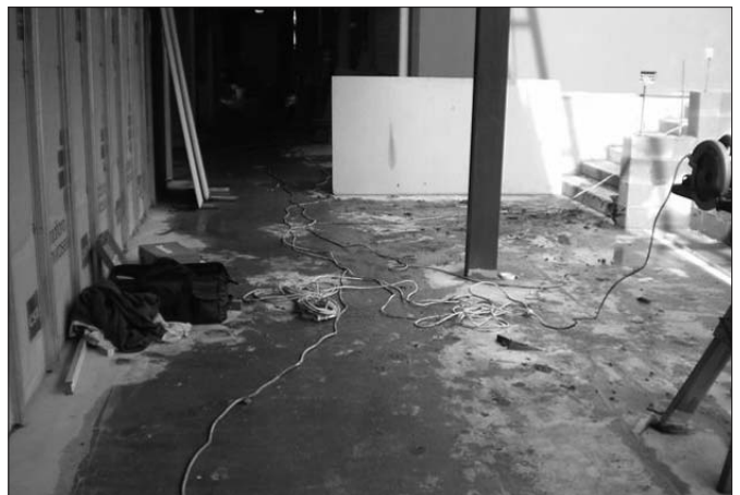
Leads trailing in wet mud show a complete disregard of AS/NZ 3000 and 3012 standards — too often found on this builder's sites.
