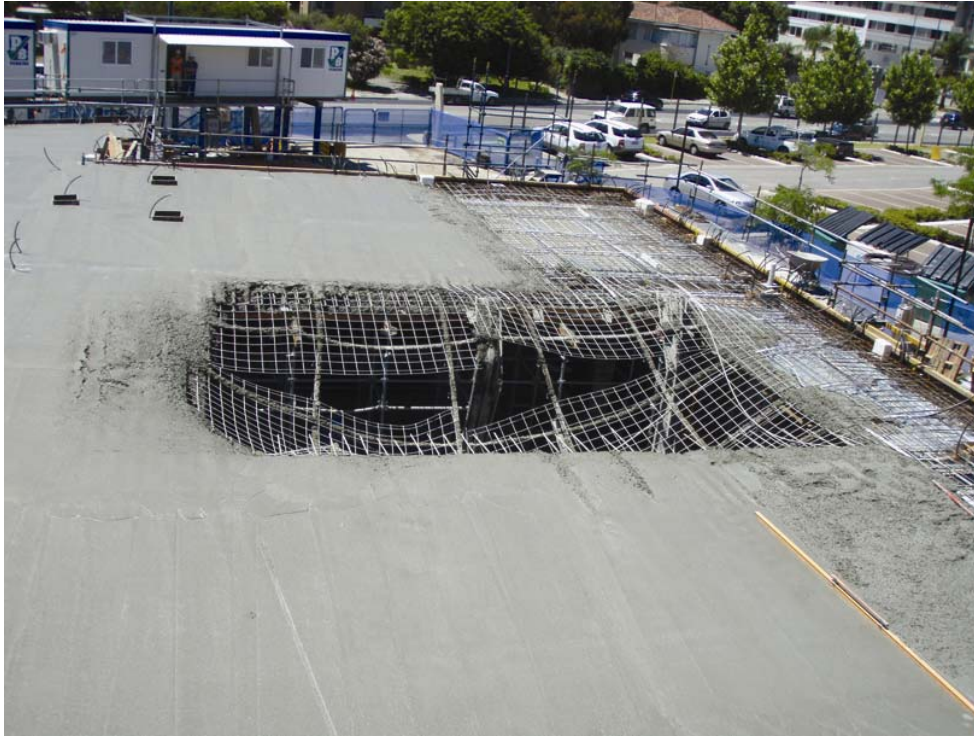
Collapsed formwork leaves large hole. Notice where concreter's screed is located.
