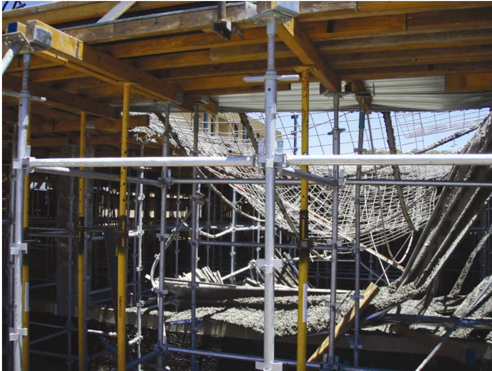
Notice the concreter's screed in the centre of the collapse
