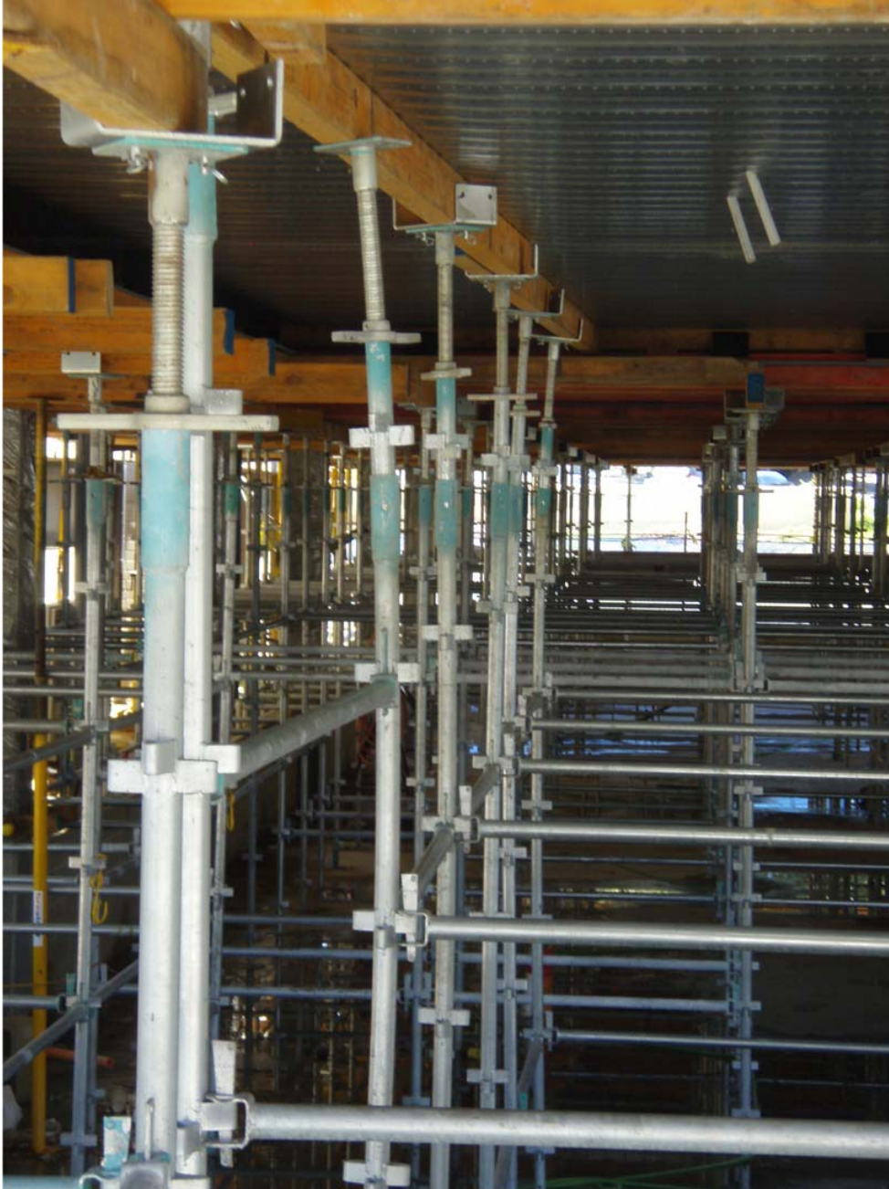
Scaffold standards buckling under the pressure from concrete above. Notice the distance between jacks and bottom ledgers.
