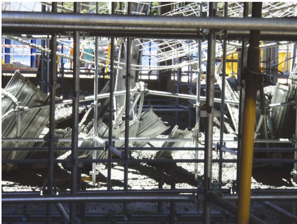
Twisted formwork scaffolding standards
