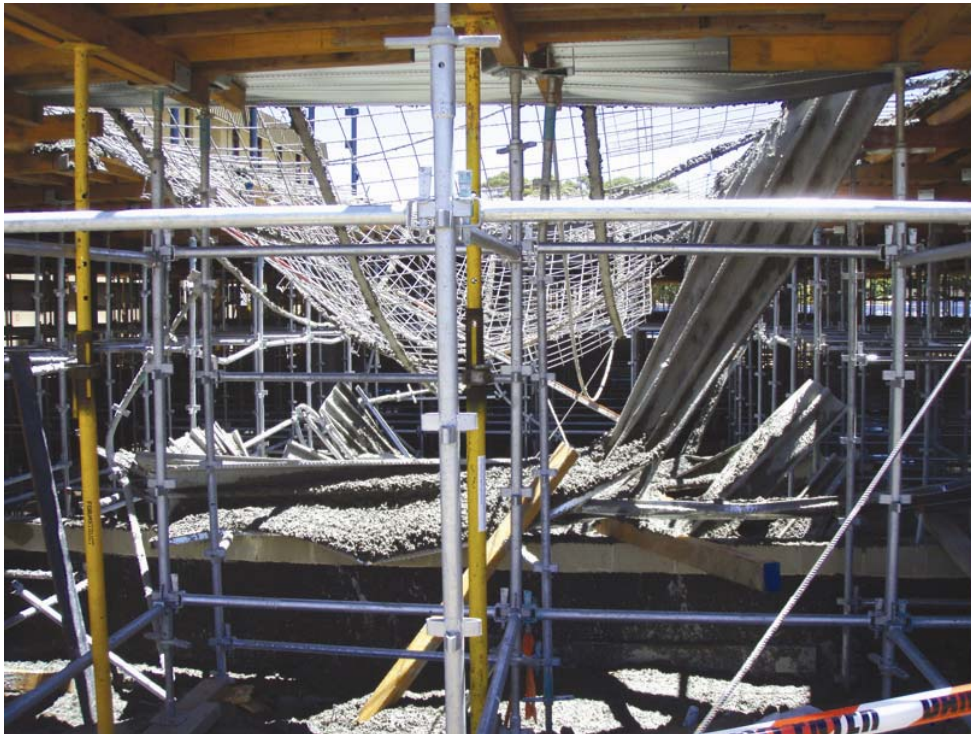
Collapsed bond-deck and post tension cables
