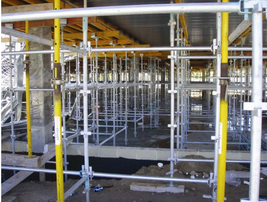
No bracing throughout star-sure formwork system
