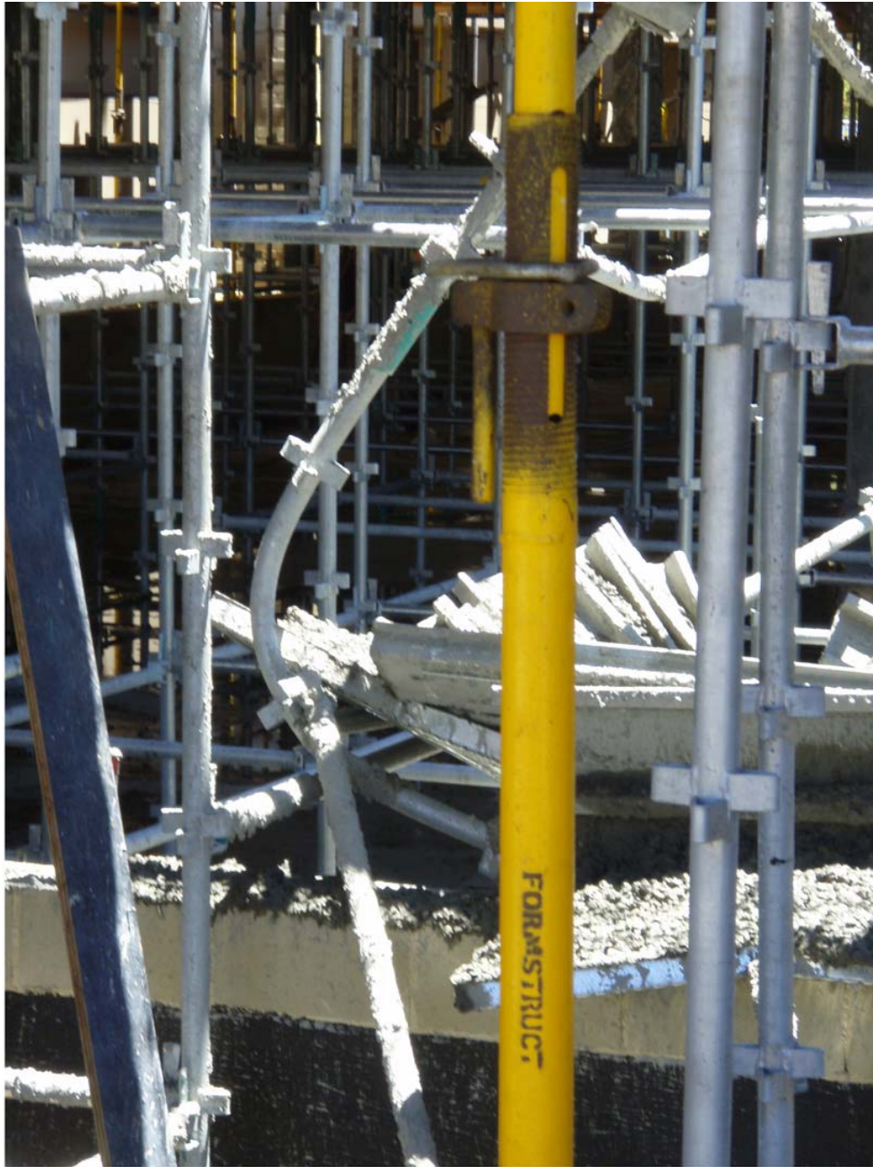
Twisted star sure scaffold components
