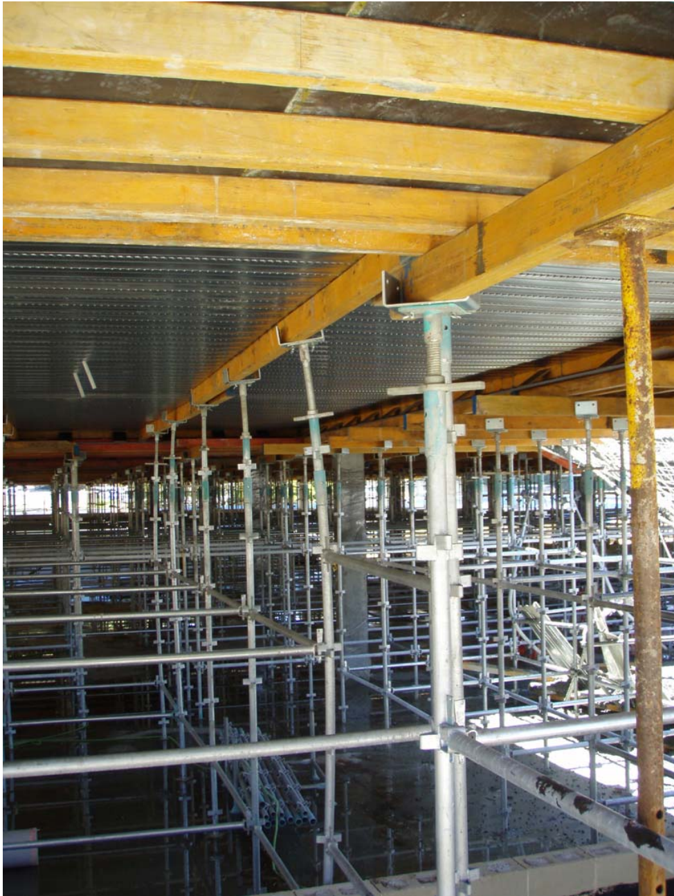
Scaffold standards buckling under the pressure from concrete above. Notice the distance between jacks and bottom ledgers.
