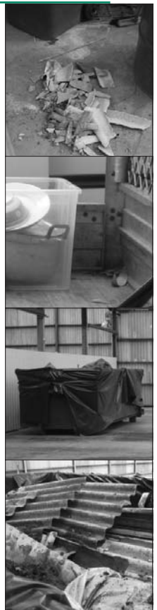
Top 1. Asbestos heap not far from drain.
