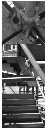
Above: the temporary rectification with doubles and clips; open rises allow the wind to blow through; enclosed stairs which caused problems in strong winds.
