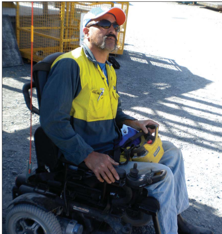
Joe Salu operating a self-erecting crane from his electric wheelchair and setting new goals for the future.
